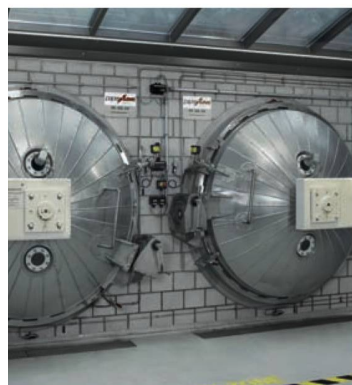
Papersave swiss plant, Wimmis. Both chambers are closed. The plant is in operation.
