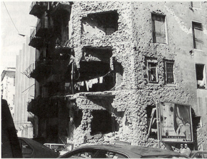
Severe damage was done to these buildings in Beirut, Lebanon, after a massive air attack by the Israeli Air Force.
