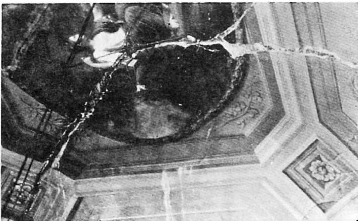
Pic.21: Cracks in the vaults of Ducal Palace of Modena
