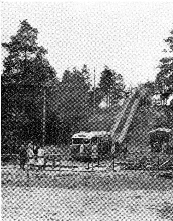
FIG. 5. Slope provided with runway of wood. In the foreground, the parapet fixed in the concrete foundation.
