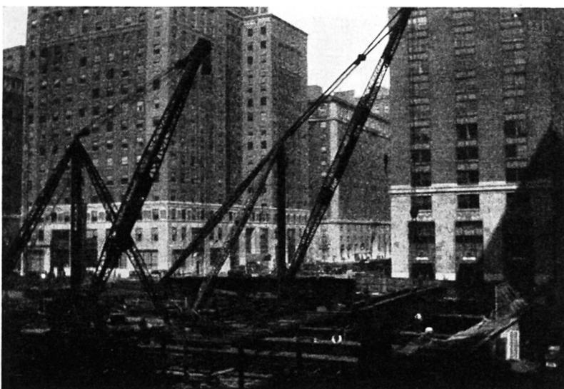
Fig. 14. Stiffleg derricks are sometimes used as travelers to erect heavy steel below street level, then setting up guy derricks for the upper, lighter structure.
