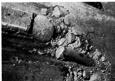
Fig. 5. The Fatigue Rupture of the Connector. The Picture Shows the Concrete Slab, Upside Down, with the Connector Ends, After Failure.
