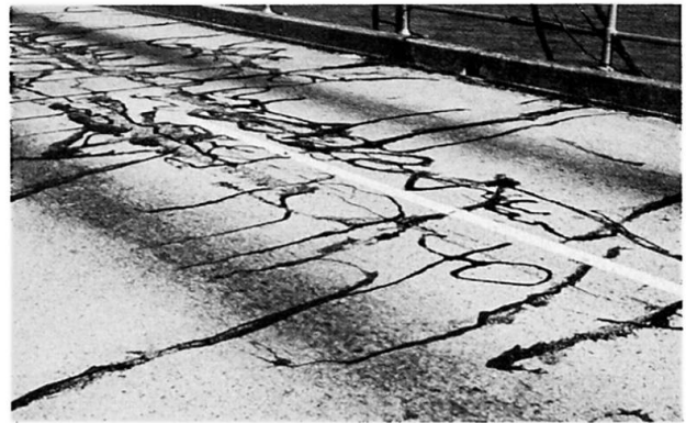
3. Deteriorated riding surface temporarily repaired with poured asphalt
