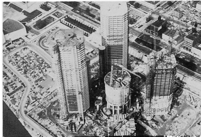
DETROIT RENAISSANCE: This is a very large and complex project consisting of a 70-story concrete structure hotel, four 39-story steel structure office buildings connected with a 7-story concrete podium for parking and commercial space.
