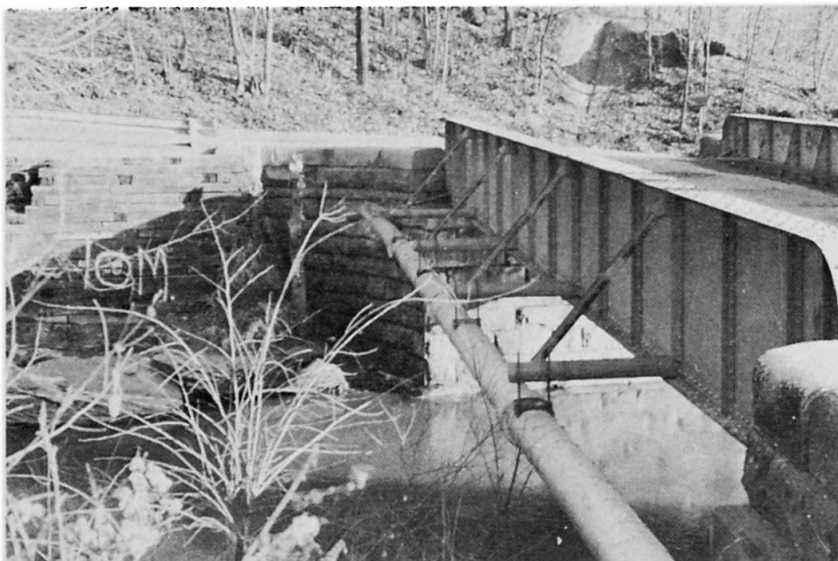
Photograph 3: Case Study 2 - Deteriorated steel through-girder bridge.
