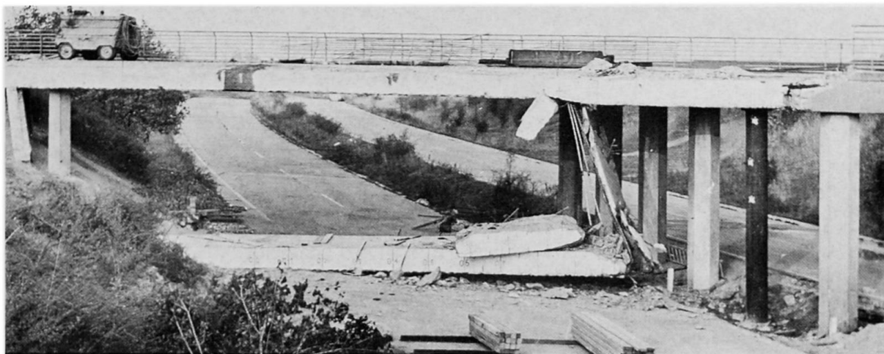
Fig. 7. The collapsed slab strip.
