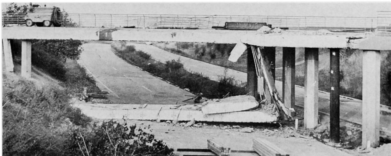
Fig. 7. The collapsed slab strip.
