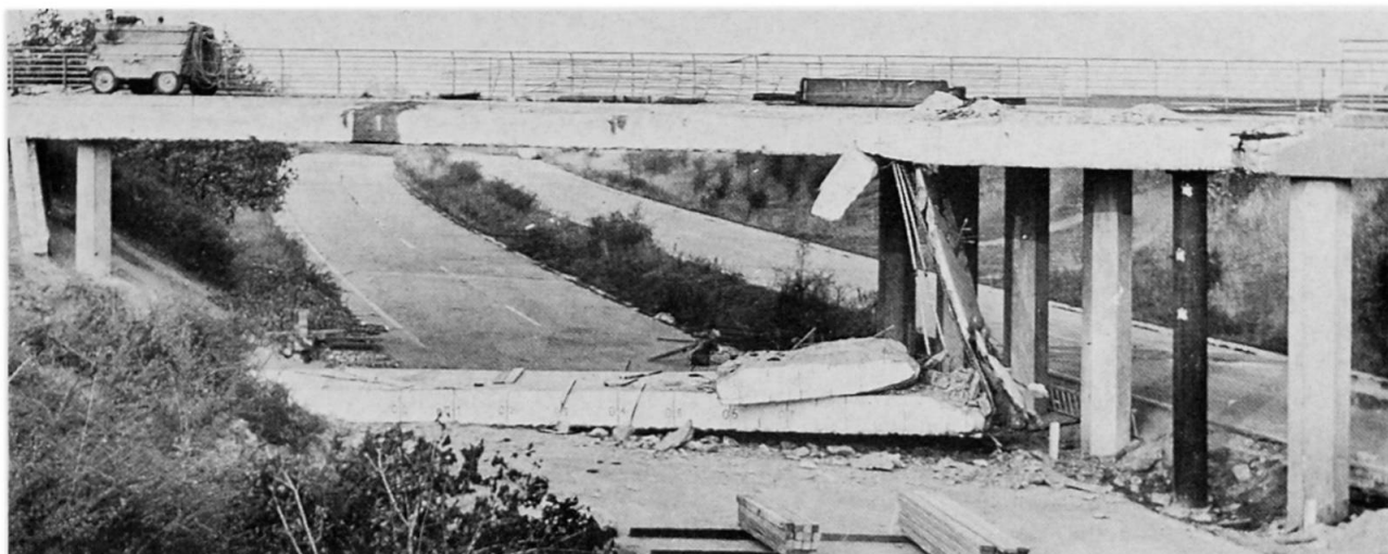
Fig. 7. The collapsed slab strip.
