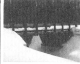
FOX LAKE Bridge New prestressed laminated wood rigid frame. Built 1981, Sudbury, Ontario.
