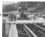
VICTORIA ISLAND Bridge. Deck replacement with prestressed wood panels. Ontario Hydro Ottawa, 1984.
