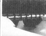
FOX LAKE Bridge New prestressed laminated wood rigid frame. Built 1981, Sudbury, Ontario.
