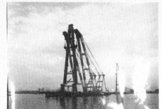
A-frame towers, the height of 104 m and the weight of 1250 ton, were hoisted into place by a 3000-ton floating crane in July, 1983
