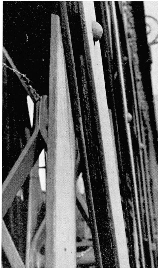
Fig. 9. Influence of design on corrosion. Difficult access to surfaces for repainting (railway bridge at Putney).
