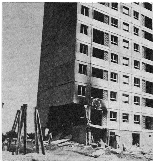
Large panel building in Algeria, Granström & Carlsson (1974). An explosion in the ground floor caused considerable damage in the panel structure without damaging the elements above.
