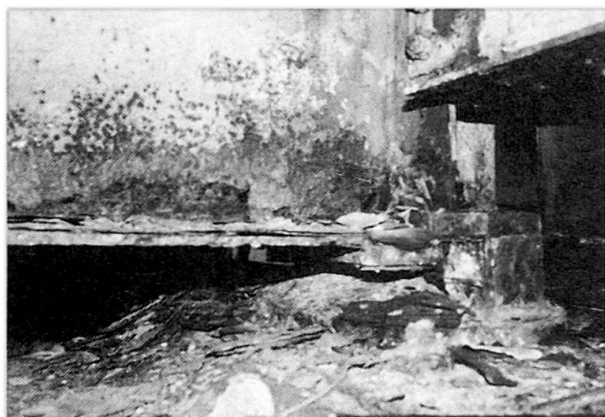
An example of corrosion
