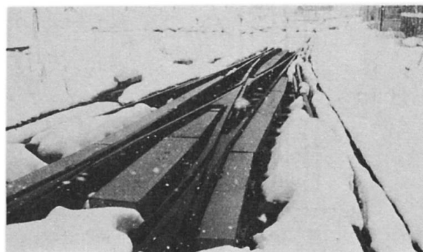
Photo 2 Snow melter for turnout
