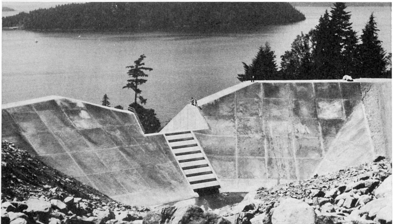
Fig. 1 Fill type debris barrier
