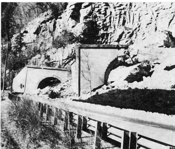
Fig. 1 Tunnel portal destroyed by rock slide
