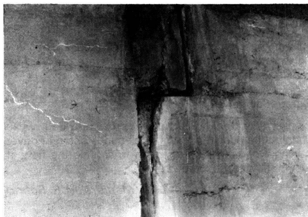
Fig. 1 Distress at articulation
