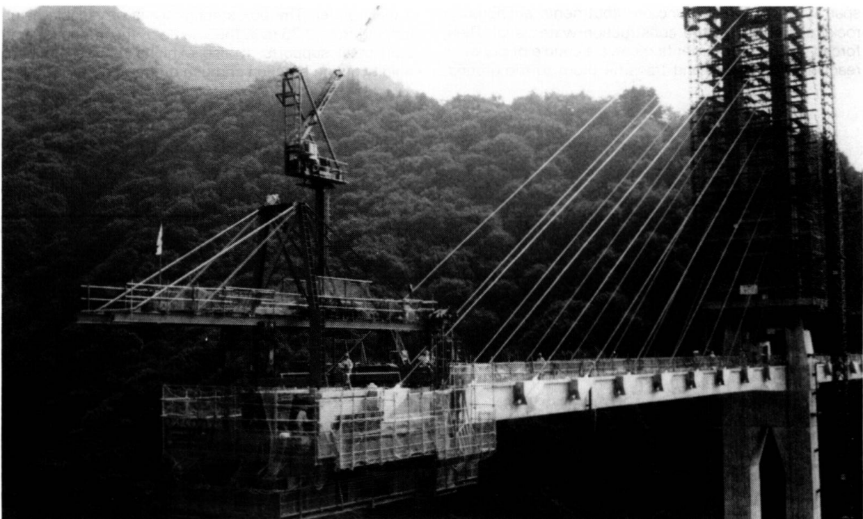
Fig. 4 View of the Suspended Long Traveller (SLT)
