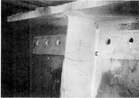
Fig. 11 Hole at Stiffener
