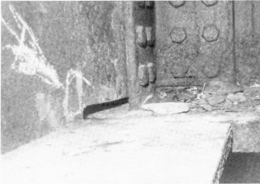
Fig. 5 Vertical and Horizontal Fatigue Cracks at Bottom Web Cope
