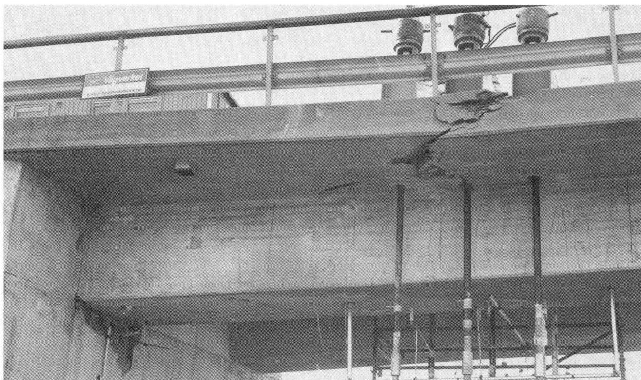
Fig. 7 Failure in the prestressed bridge. Cracking, support failure and concrete compression failure at the top of the loading section can be seen.
