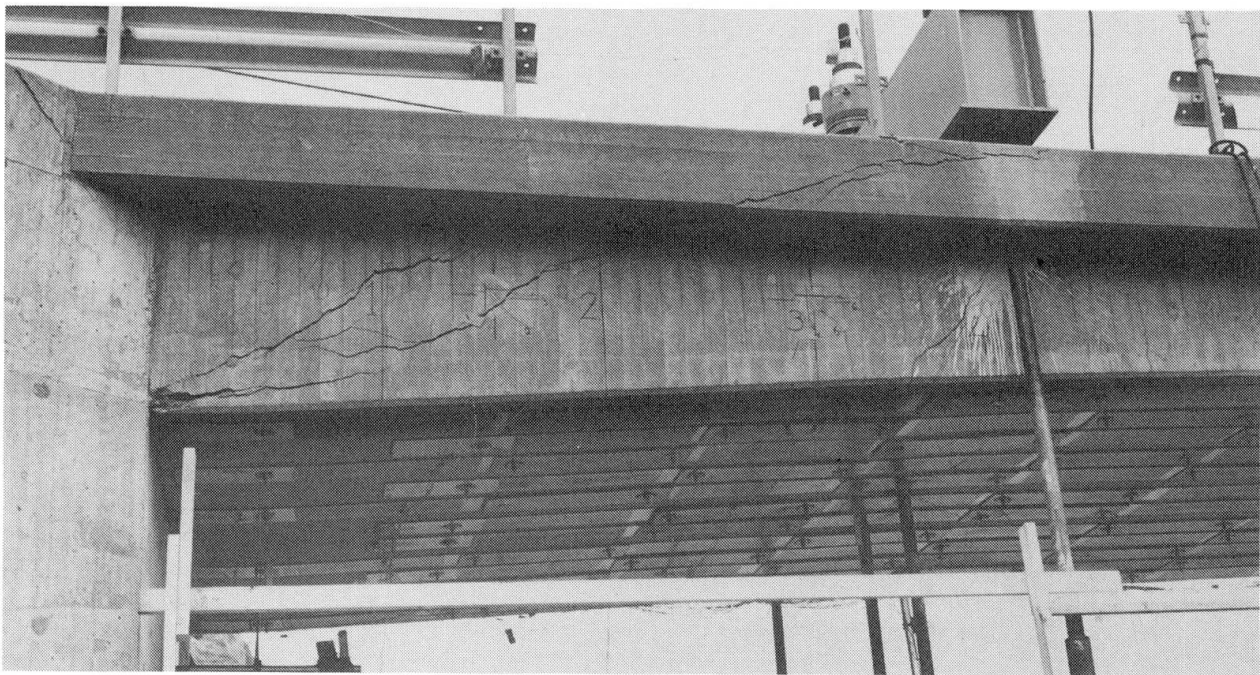
Fig. 6 Shear failure in the non-prestressed bridge
