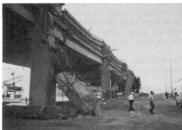
d) PHOTO OF COLLAPSED STRUCTURE
