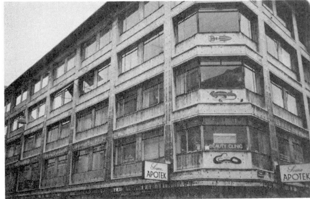
Figur 4: Miscoloured facade due to dirt and soot
