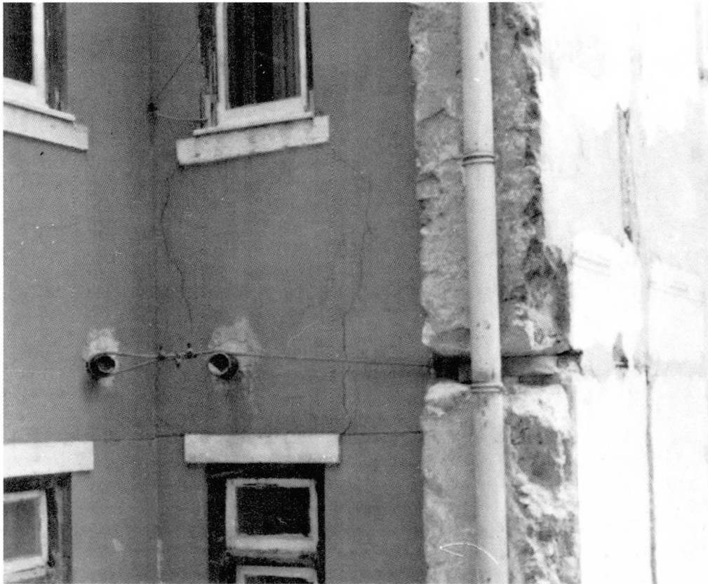
Fig. 2: Damaged masonry wall due to demolition of an adjoining building
