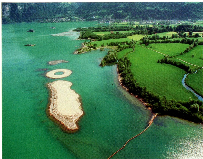
Filling with excavated material from the Gotthard in the Reuss delta near Flüelen.
