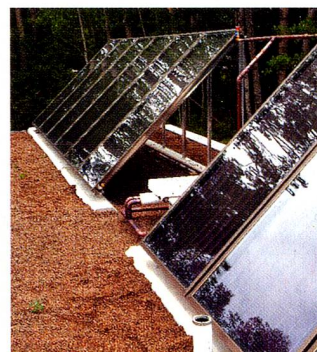
Solar panels which are part of a sophisticated solar hot-water system that meets the high volume hot-water needs of Waldsee BioHaus.
