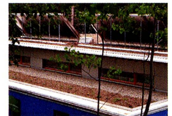
Extensive green roof of Waldsee BioHaus that serves to retain rainwater, reduce the risk of erosion and act as a heat buffer during the summer.
