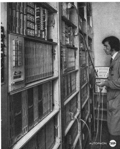
Fig. 4 Part of the installations at Zurich
