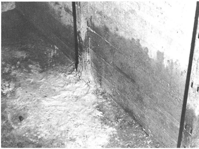
Fig. 7 Multiway duct at Egnach In this chamber, water has penetrated at the point where the steel profile has been set into the floor of the chamber, as can be seen from the lime crust formation
