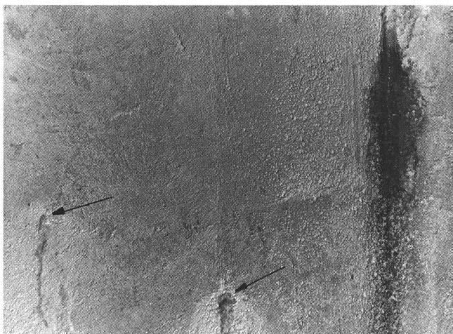
Fig. 8 Multiway duct at Egnach In another chamber, strongly basic water penetrates the concrete at two points on a longitudinal wall — marked by two arrows in the Figure
