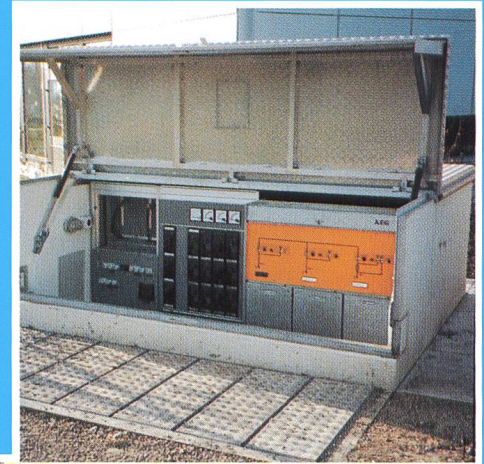
Station compacte Kompaktstation in Gossau/ZH
