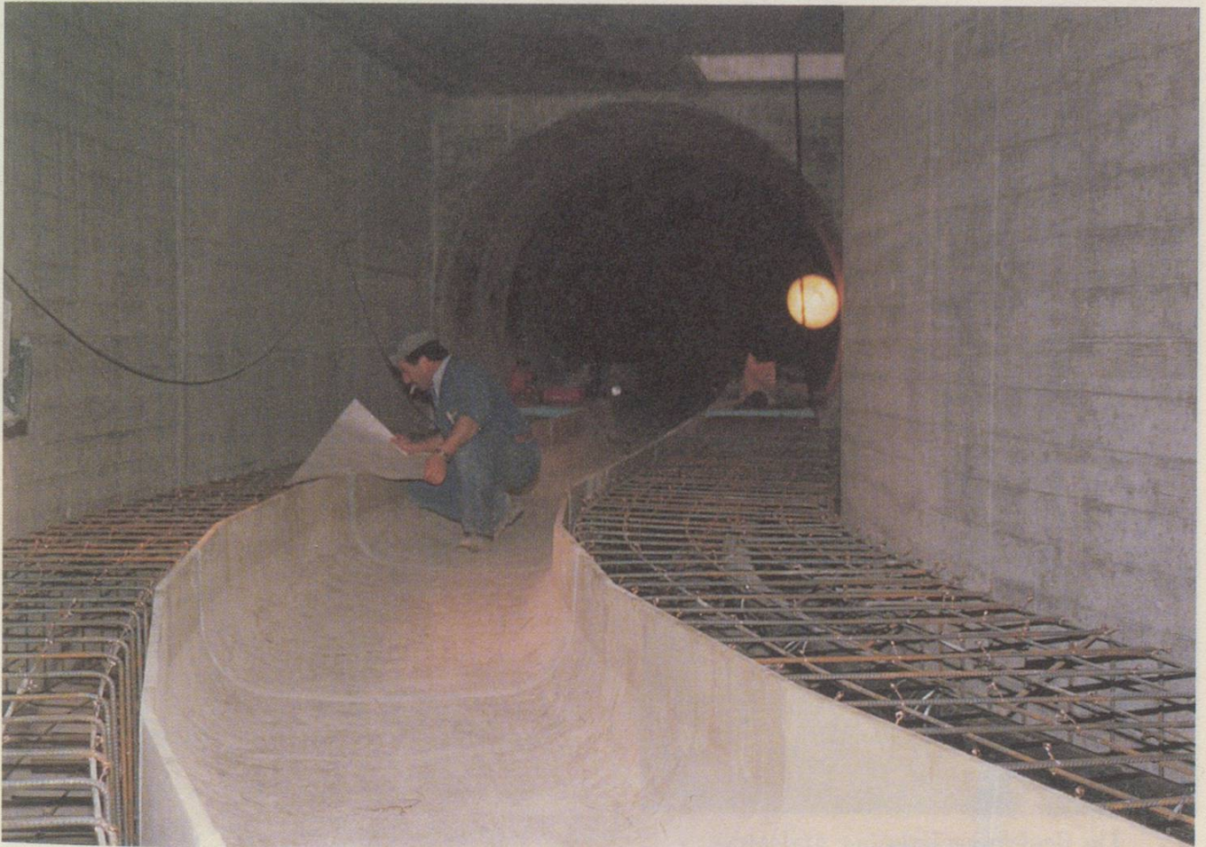
Construction of the tunnel at the site of the new power plant.
