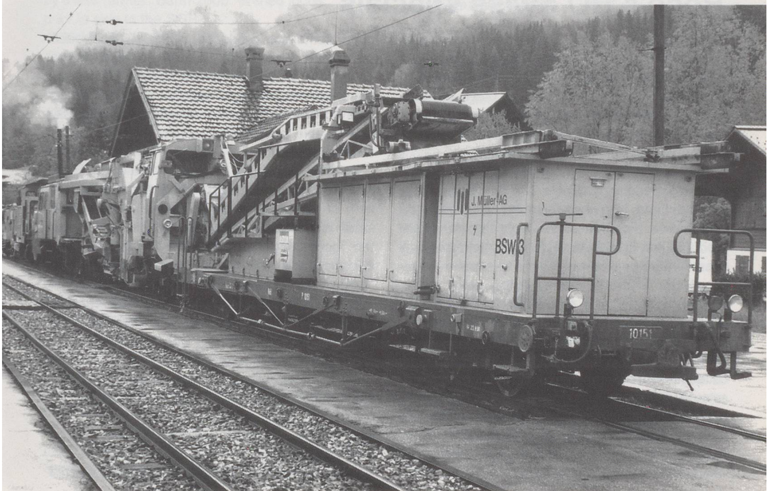
Below: The ballast cleaning and replacing train waits to follow on behind when the track crews have finished.
