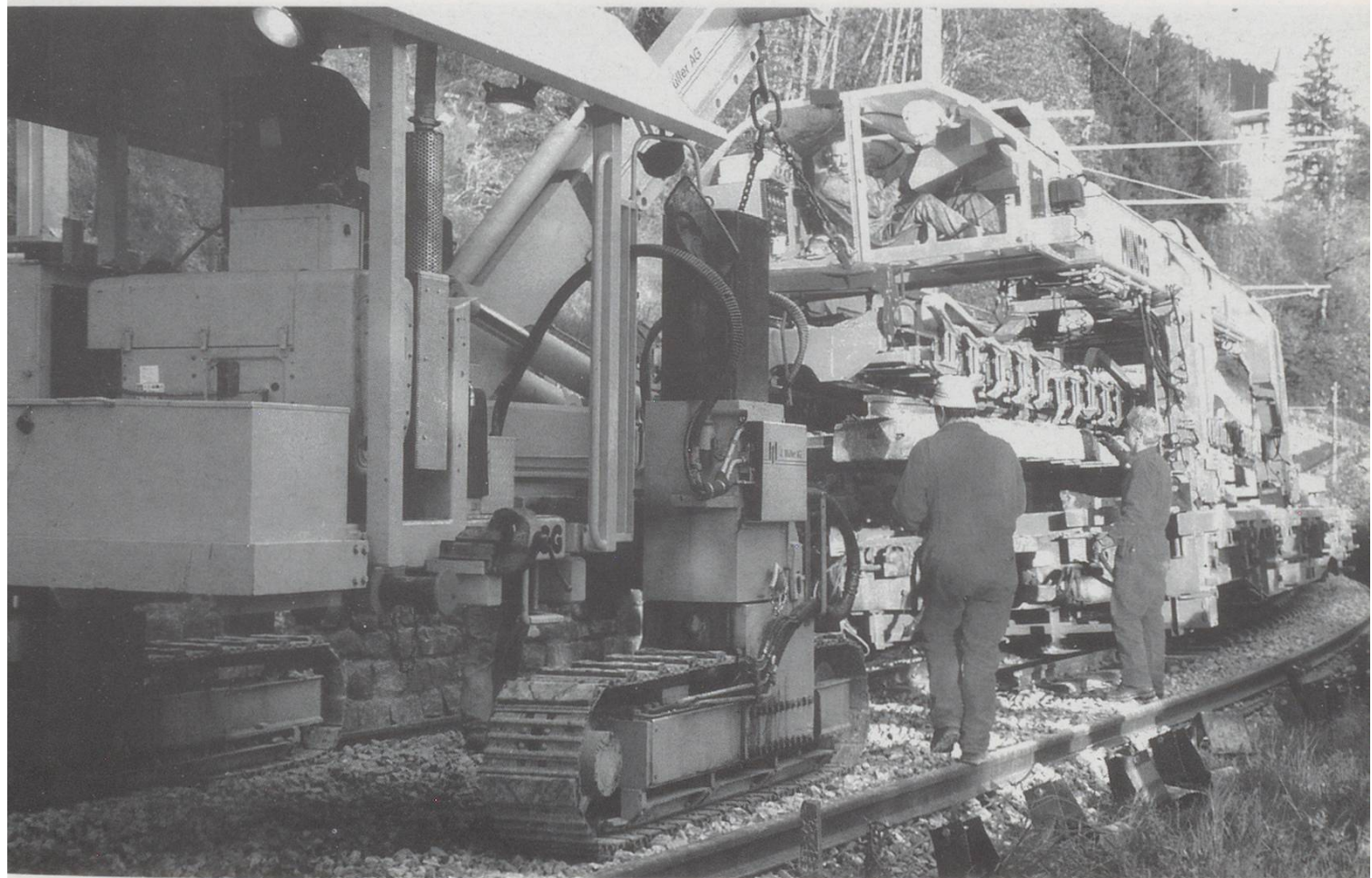
Below: A clear view of the tracked crane manoeuvring the spar under the wagon crane, the driver of the wagon crane is visible above spar in a semi-lying position, access is via the glass doors.
