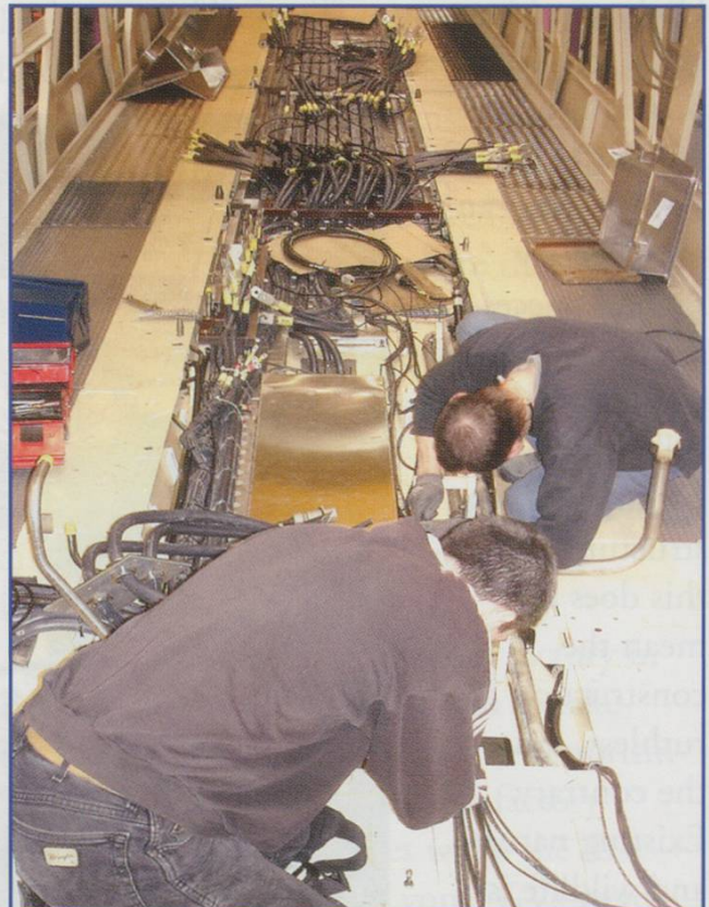
Two technicians are installing cables into channels in the floor. Each cable is tested as soon as it is connected.
