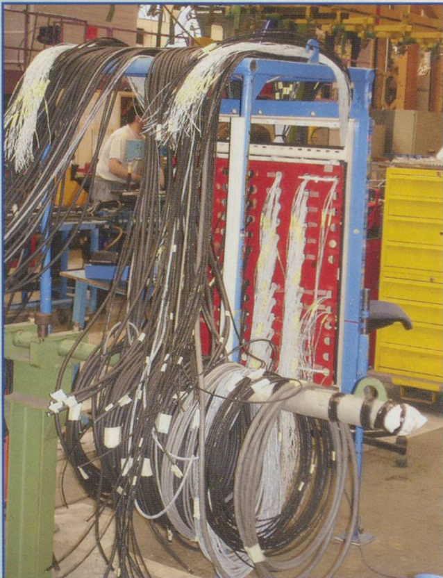
The stock needs many miles of cables. Here some hang on the parts trolley: each one is pre-cut to the required length and labelled. The yellow trolley on the right is for tools - nothing is left lying around.
