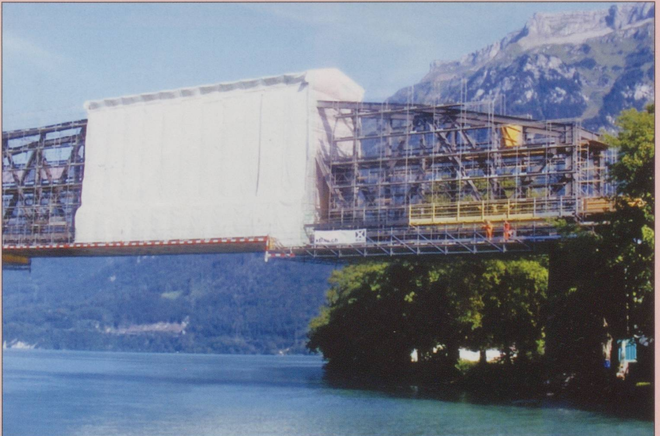
Repairs to ZentralBahn bridge over the end of Lake Brienz at Interlaken. PHOTO: Alan Pike
