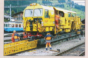
Unloading a track maintenance machine at Zweisimmen from the standard to meter gauge. PHOTO: Roy Marriott
