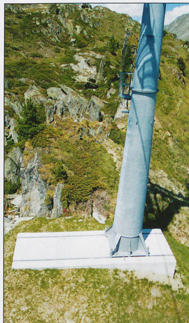
HEADER PHOTOGRAPH: The top station for the Aletsch Glacier cable car.
