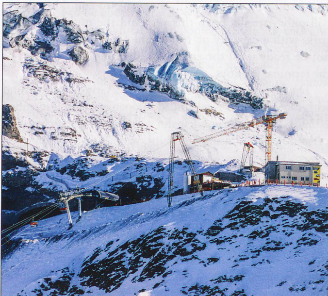
TOP: Grindelwald Grund construction site. The new base station of both the GGM and EigerExpress.
