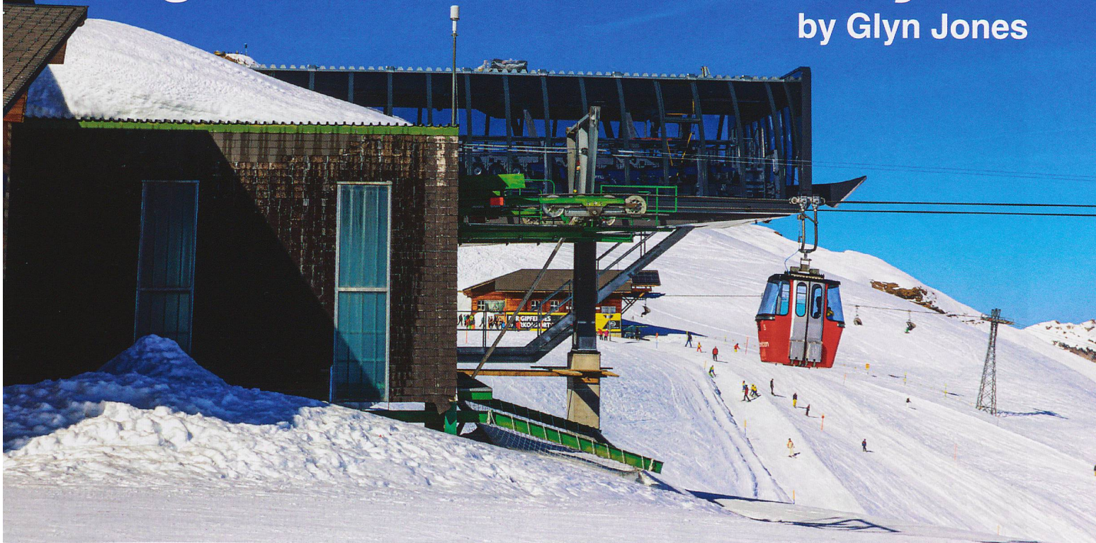
Old and new – side by side. The last few days of the original Männlichen Gondelbahn with the new top station ready to take over.
