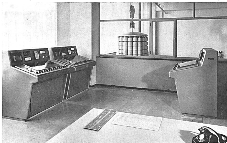
Automatic dyeing control room; in the foreground, the perforated card which commands all the operations undergone by the bobbins of yarn. The whole process is automatically commanded by remote control from 3 control desks visible in the foreground. From his control post, the operator supervises the dyeing room and the laboratory for the preparation of the dyes. (Stoffel Ltd.)
