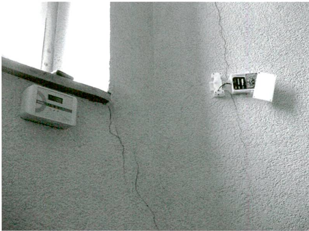
Fig. 15: Easy Crack Monitor System®.
