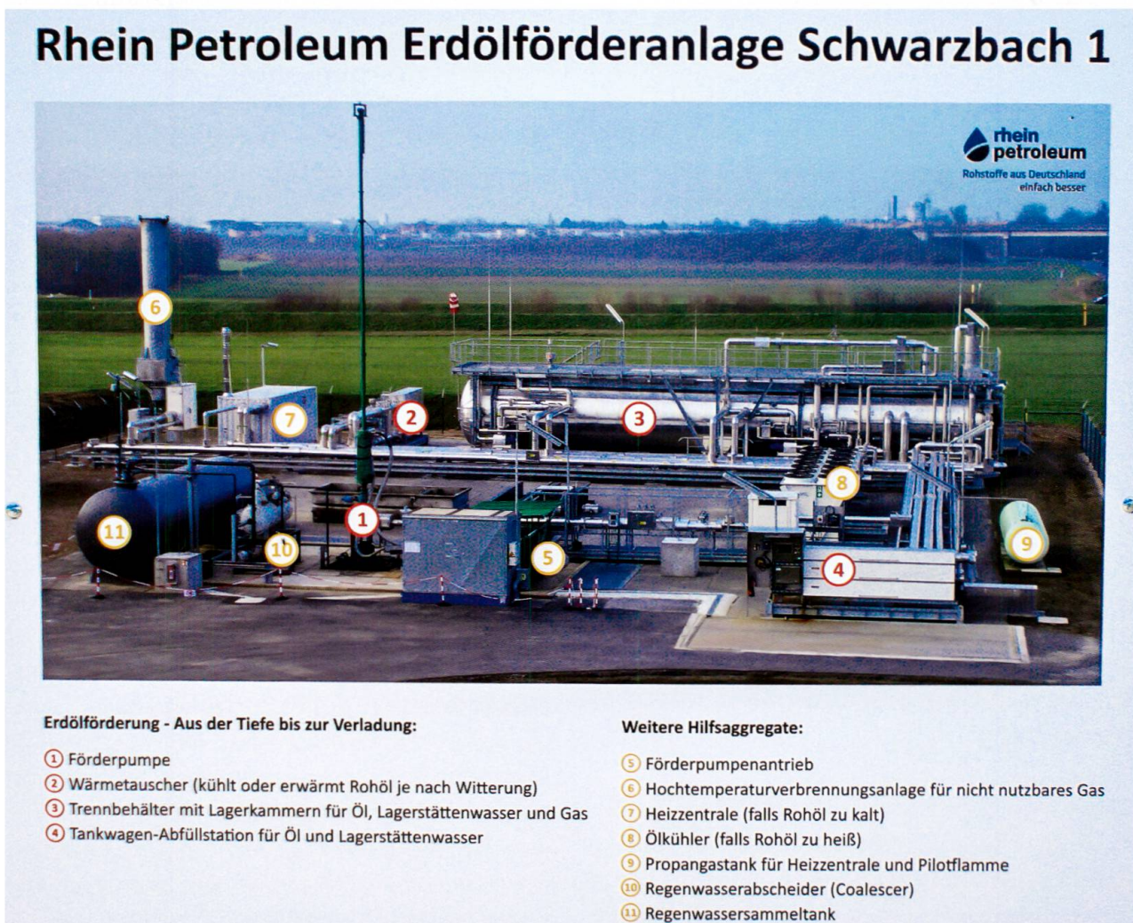
Fig. 1: Rhein Petroleum's Schwarzbach 1 oil production facility (Photograph: P. Reichetseder).
