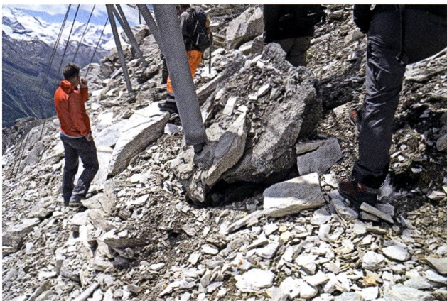
Fig. 4: Misaligned and damaged row of avalanche defense snow nets in a permafrost talus slope at Wisse Schijen (Randa, Canton Valais), resulting from differential downslope deformation and subsidence of the active layer.
